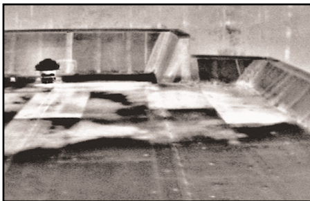
SuperiorScan's Thermal Inspection discovers insulation moisture problems.
